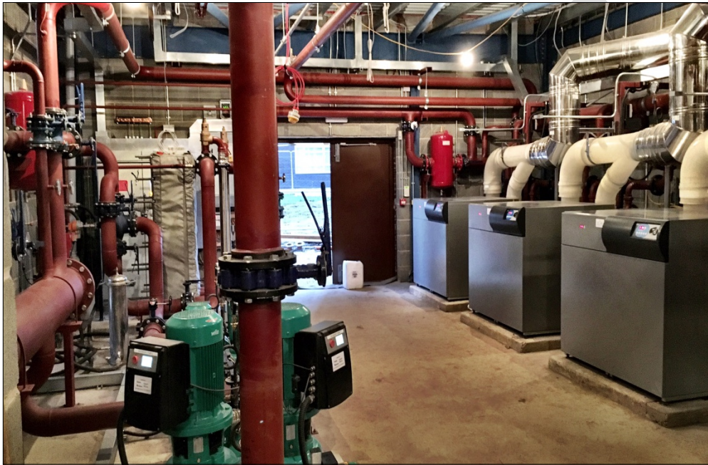
Biomass energy centre, serving Clyde Court, Clyde Grange and Phil May Court flats.
